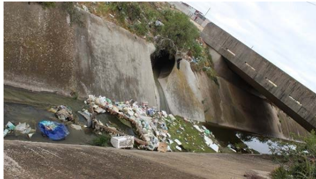
Photo: Motherwell storm water canal
